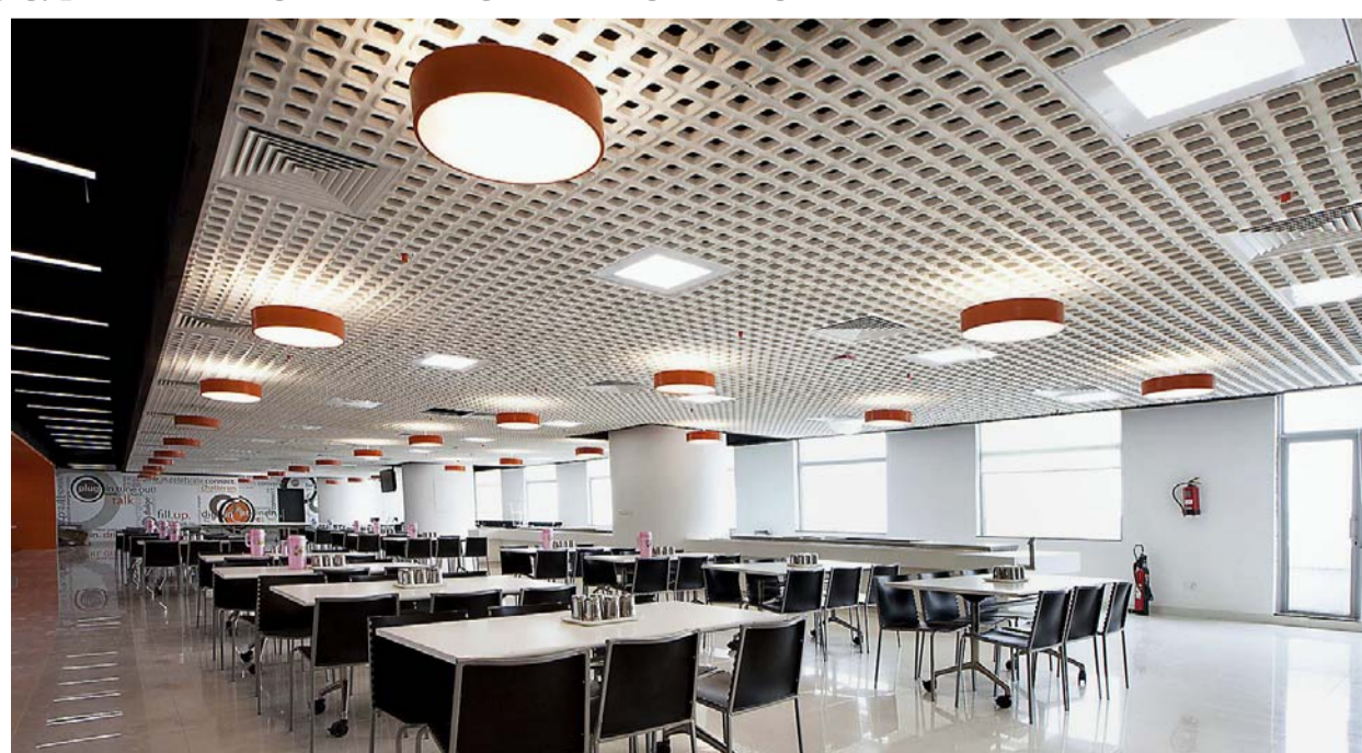
MAJOR PROBLEM: The biggest problem with false ceilings is sagging and staining.
